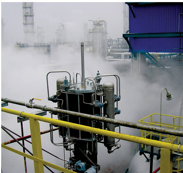
Figure 1. Masoneilan control valve with digital valve positioner.
